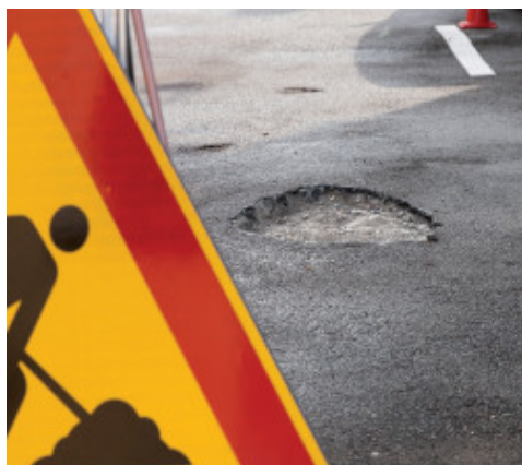
Road in a hole ready to be repaired
